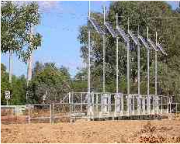
Seven solar panels operating this irrigation system
