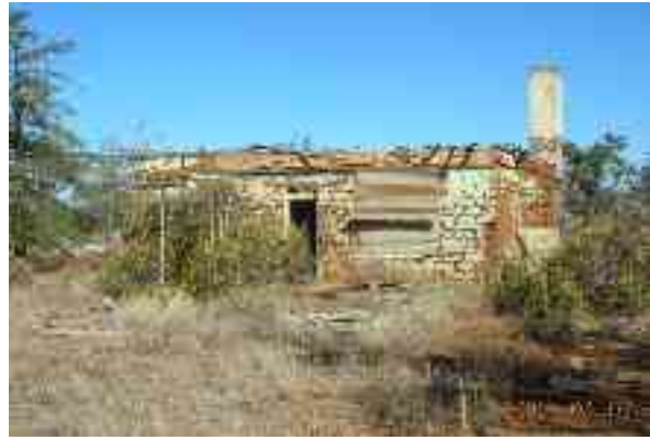
A derelict house
