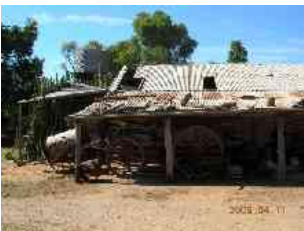
Cacti through the roof
